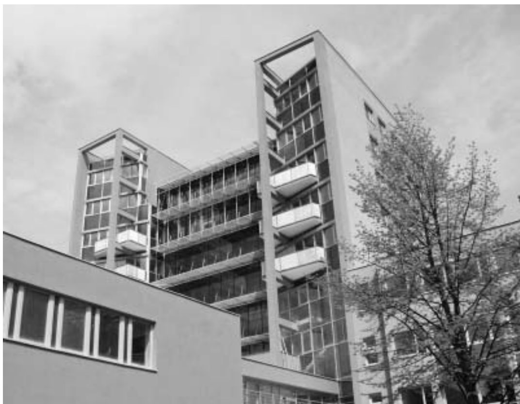
In the course of the year 2003, intensive construction works were underway at the university complex in Jižní Svahy in Zlín. The new complex for 1,500 students will be opened for lessons in September 2004, and will serve primarily the Faculty of Technology.
